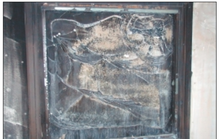
The fire resistant window effectively prevented the fire to spread
